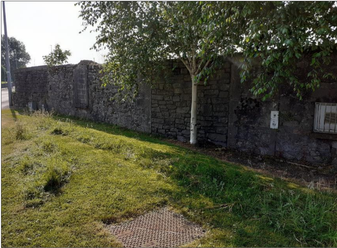
Plate 15.9: Composite wall (CH003), facing south. The wall incorporates part of a building façade, which was depicted on the 25-inch OS map (c.1900). This wall will be removed as part of the design
